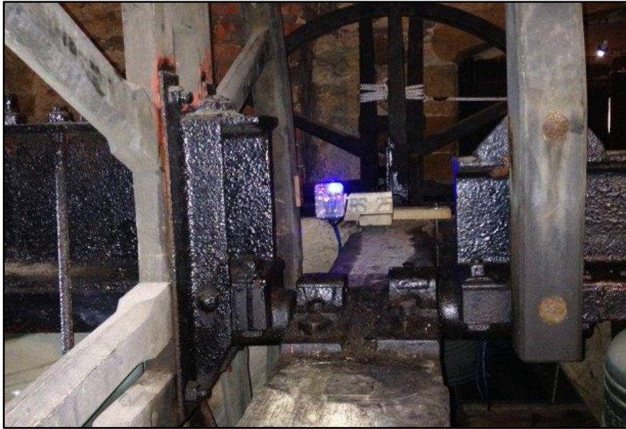
Figure 61 – Installed Sensor (Lois Weedon 6 th )
