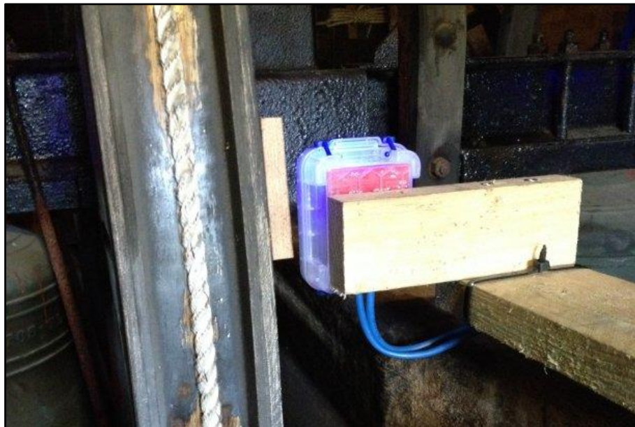
Figure 60 – Installed Sensor (Lois Weedon 4 th )
