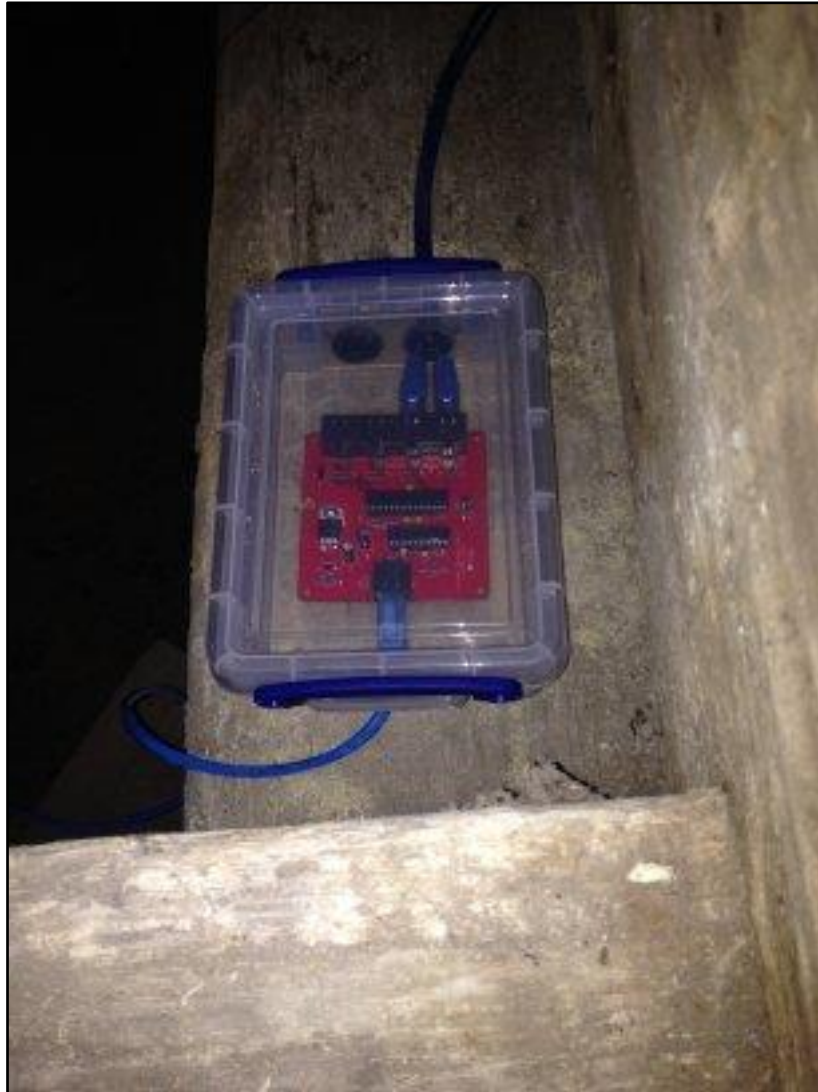
Figure 59 – Installed Simulator Interface
